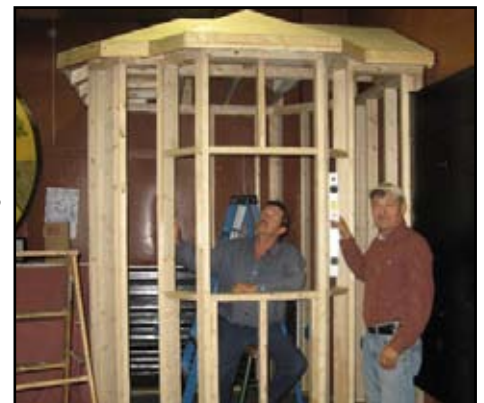
Brad Williams and Dan Felmlee inspect their work while constructing our sharp new ticket booth in the lobby of the Theatre In The Park.
